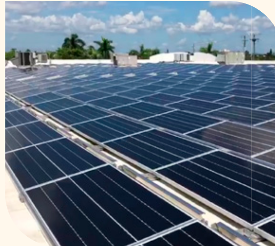
Solar Panels Distribution Center Building
